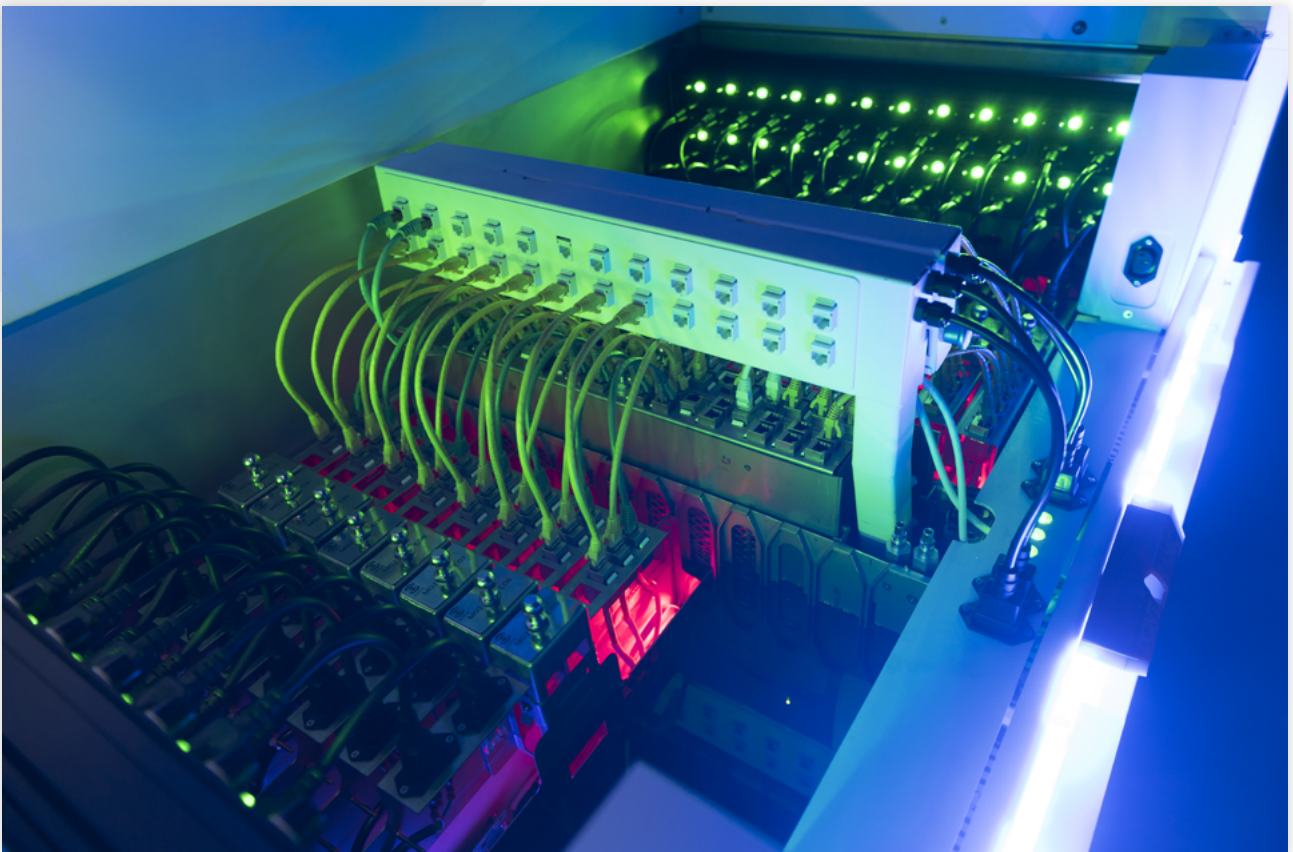
Image 1 Asperitas Immersed Computing® solution
