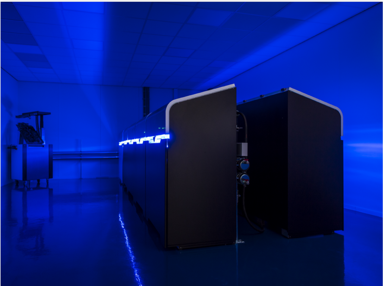
Image 3 Immersed Computing® facility
